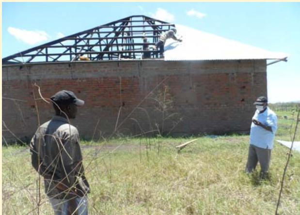
CCP dep. director Nathan Walyaula (with mask) checks on the progress of the construction.
